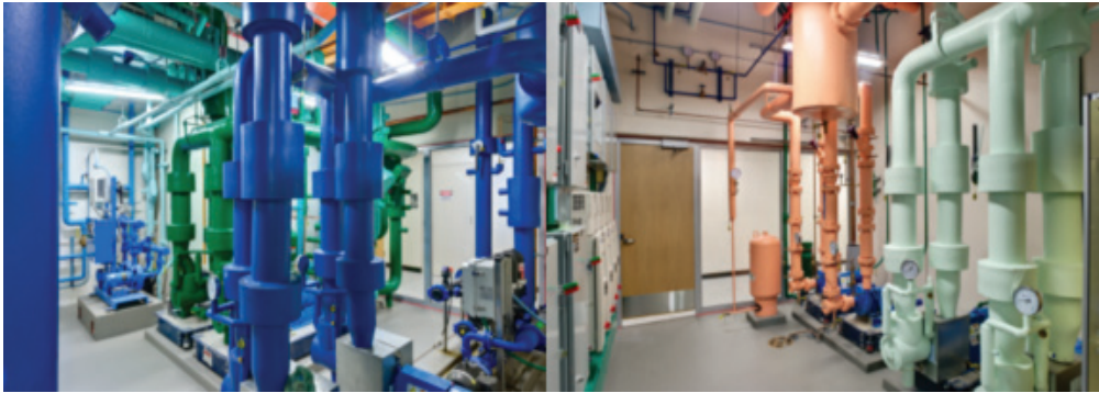
Mechanical equipment, pumps, piping, and sensors are part of the building HVAC systems. Image provided by CAKE.
