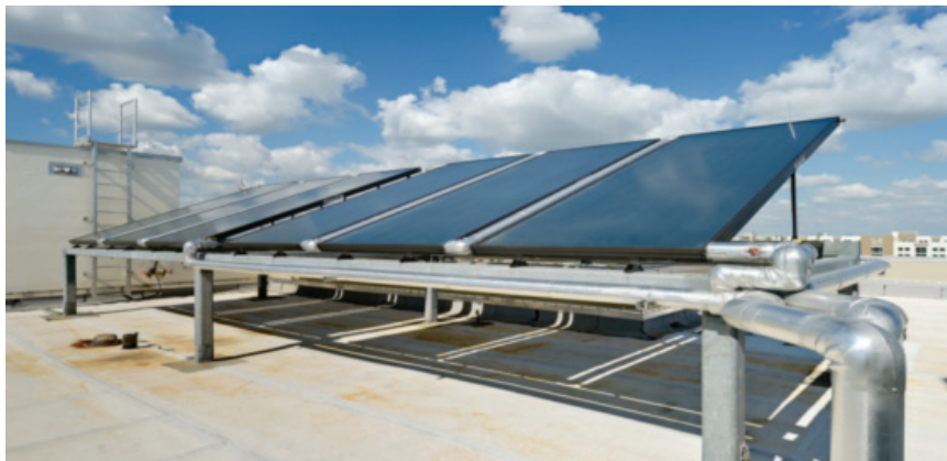
Solar photovoltaic cells on a building roof for power generation. Image provided by CAKE.
